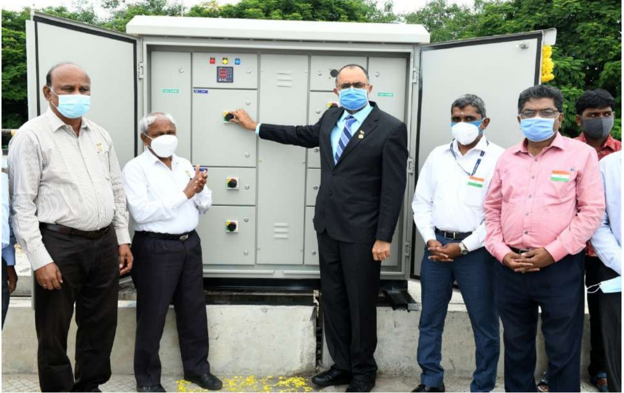
Illumination Facility at Coal Berths 3 & 4
